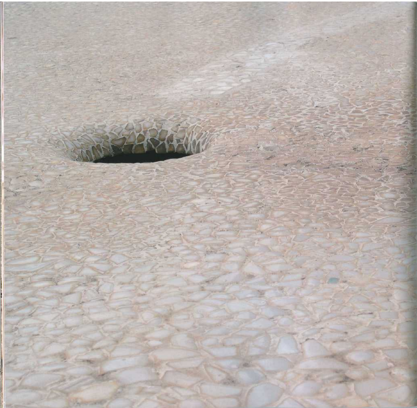
Roof drain of broken china
