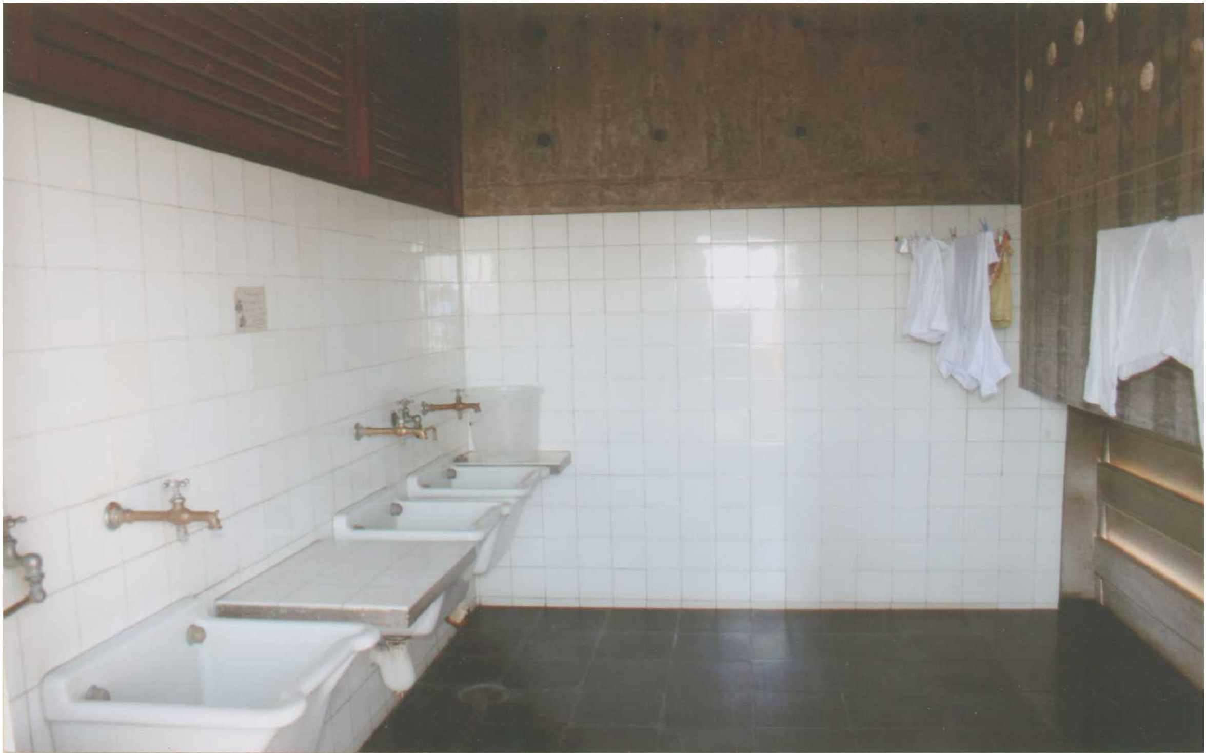
Residents' laundry room
